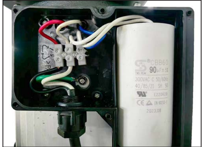
Figure 95. Motor junction box wiring.
