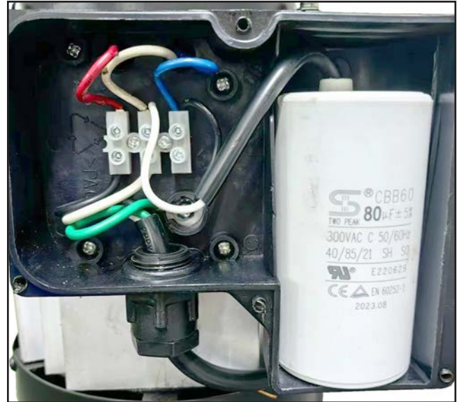
Figure 89. Motor junction box wiring.
